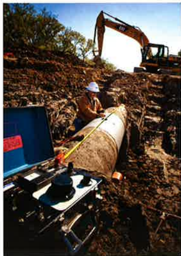
A 30-inch gas transmission line is inspected as part of our integrity management program.
