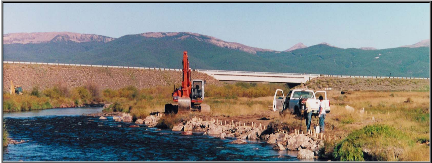
Stream bank erosion control measures and revegetation along the main stem of the Arkansas River, Summer 2000.
